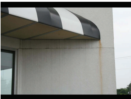
EIFS In Need of Repair
